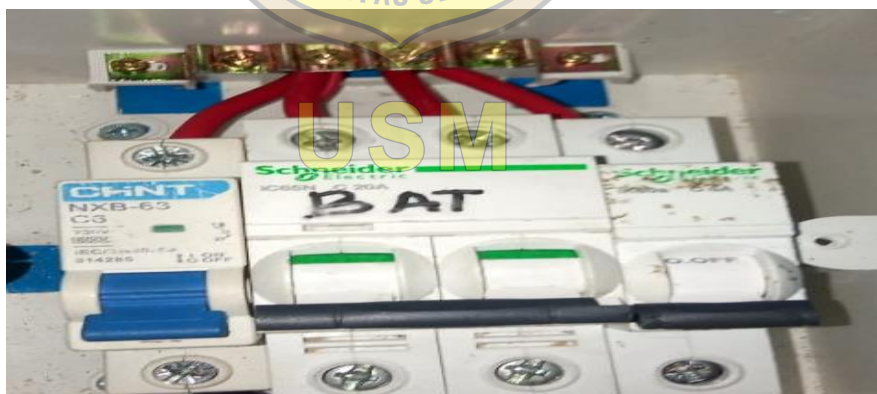
Gambar 2.7 MCB (Miniature Circuit Breaker) Schneider 20A
